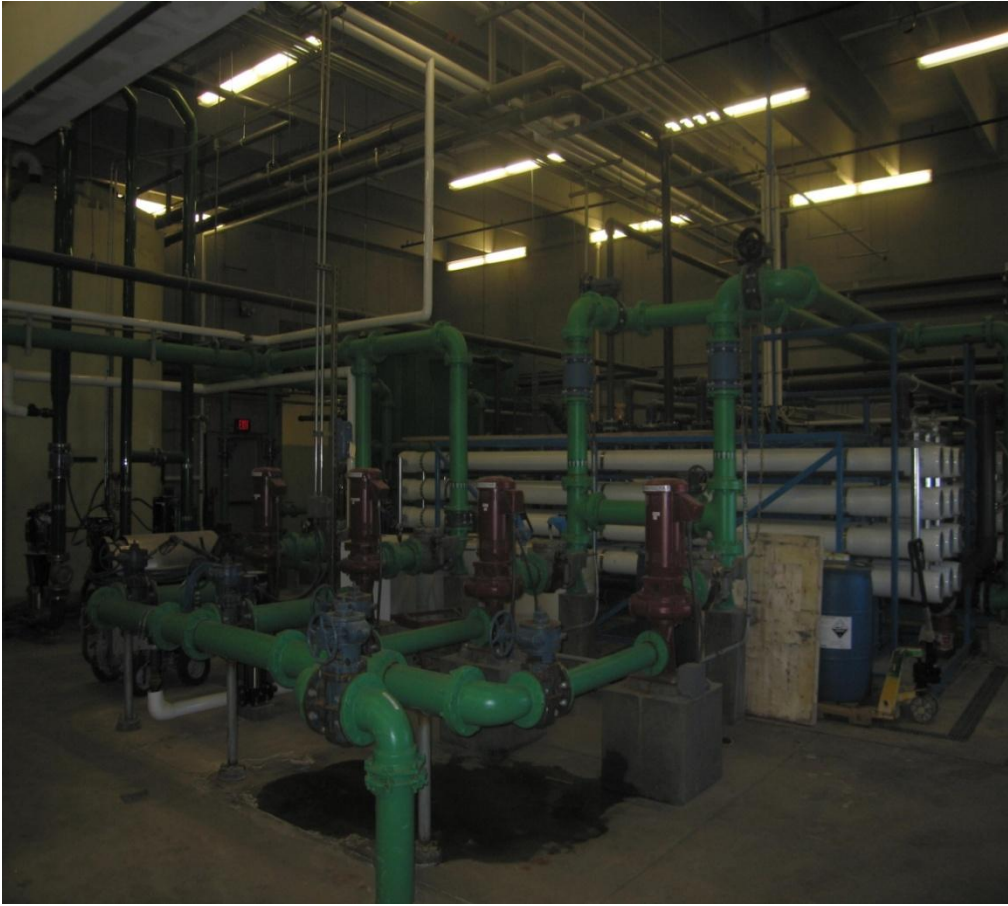
Water Treatment Piping in Water Treatment Building
