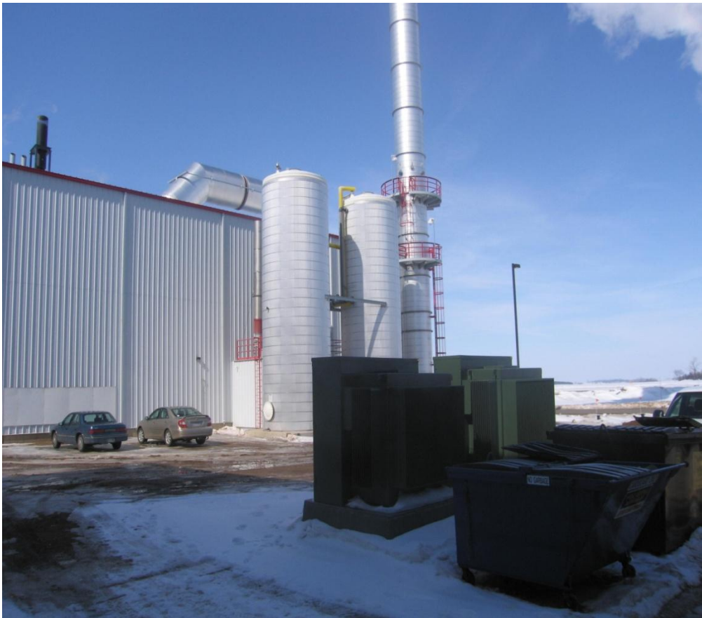
Methanators and Thermal Oxidizer Stack
